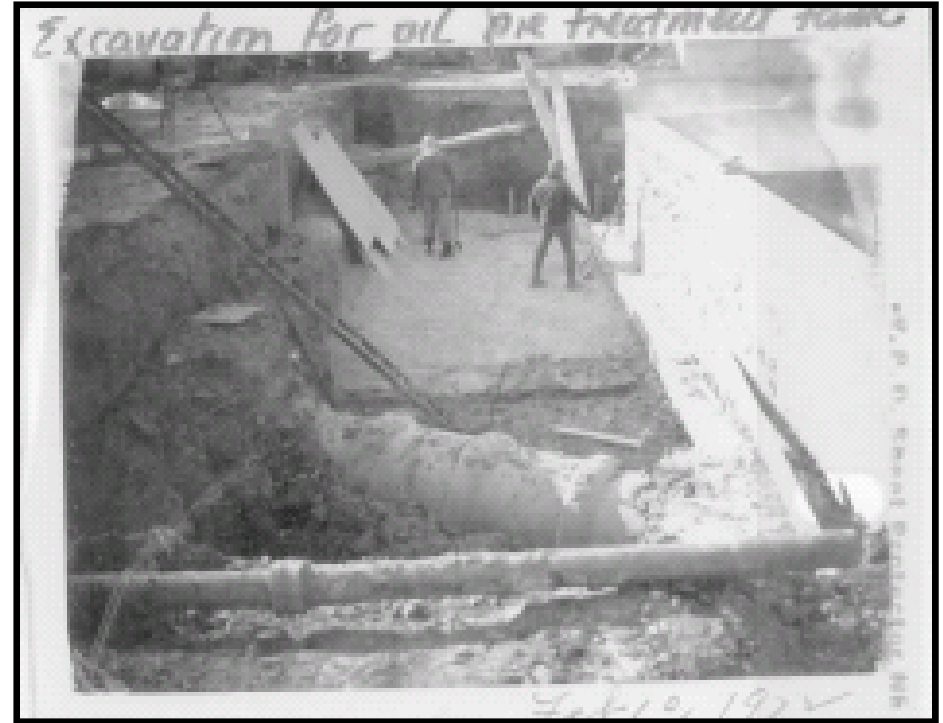
Photo 8 - February 1972 photo. View looking south from northeast corner of new Settling tanks. Note 30" diameter underground stormwater pipe and smaller sanitary pipe. Workers are standing on new base for pH adjustment tank.
