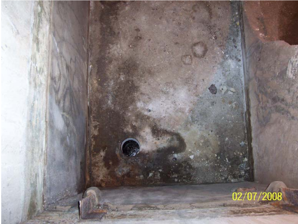
Photo 5 - Building 41, Soil boring 009 with black liquid in crushed stone sub-base.
