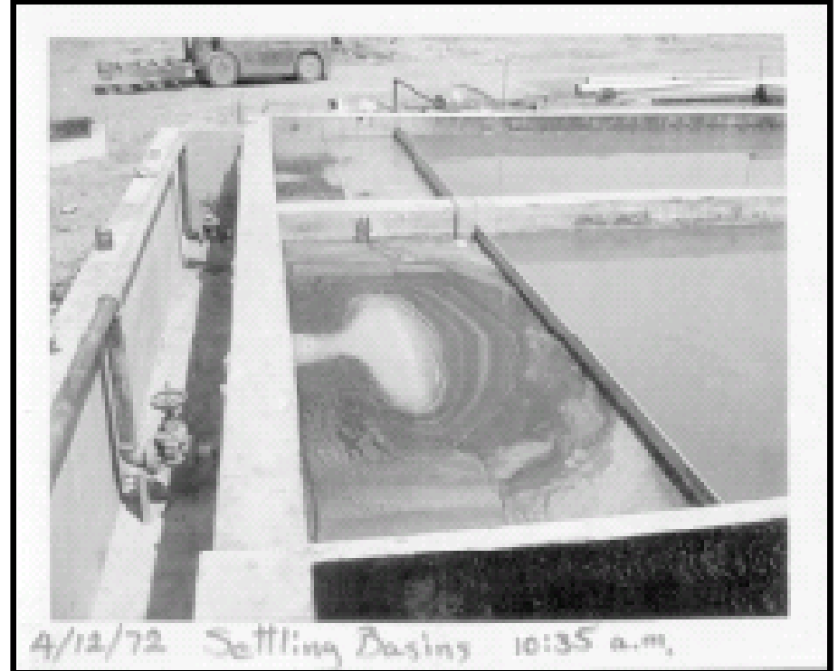
Photo 16 - April 12, 1972 photo. View looking north at west side of new settling basins.
