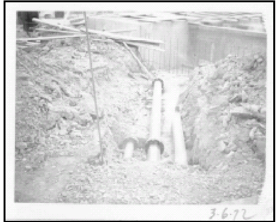
Photo 12 - March 6, 1972 photo. View looking southwest toward the northeast corner of the EQ tank. The three pipes are presumed to be from Bldg 2 WW tank area. Rebar from Neutralization tank wall construction in background.
