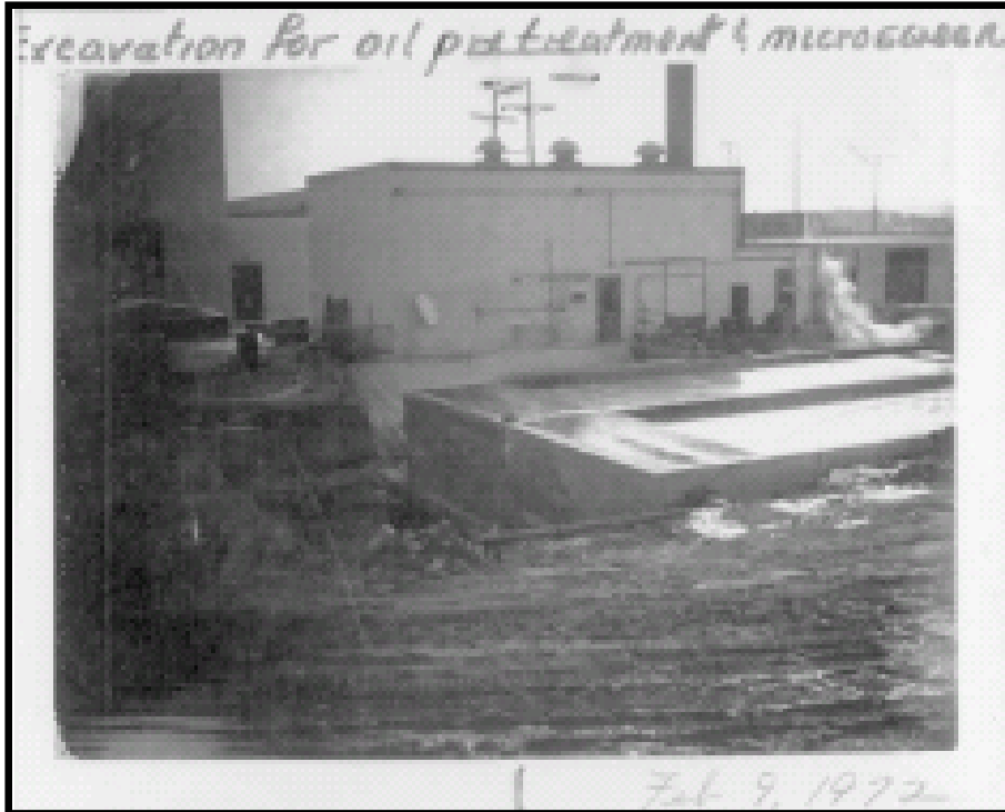
Photo 3 – February 9, 1972 photo. View looking Southwest toward north side of Bldg 41. Excavation for new EQ tank is shown in the foreground. Note that the two new settling basins have already been constructed and are filled with water.
