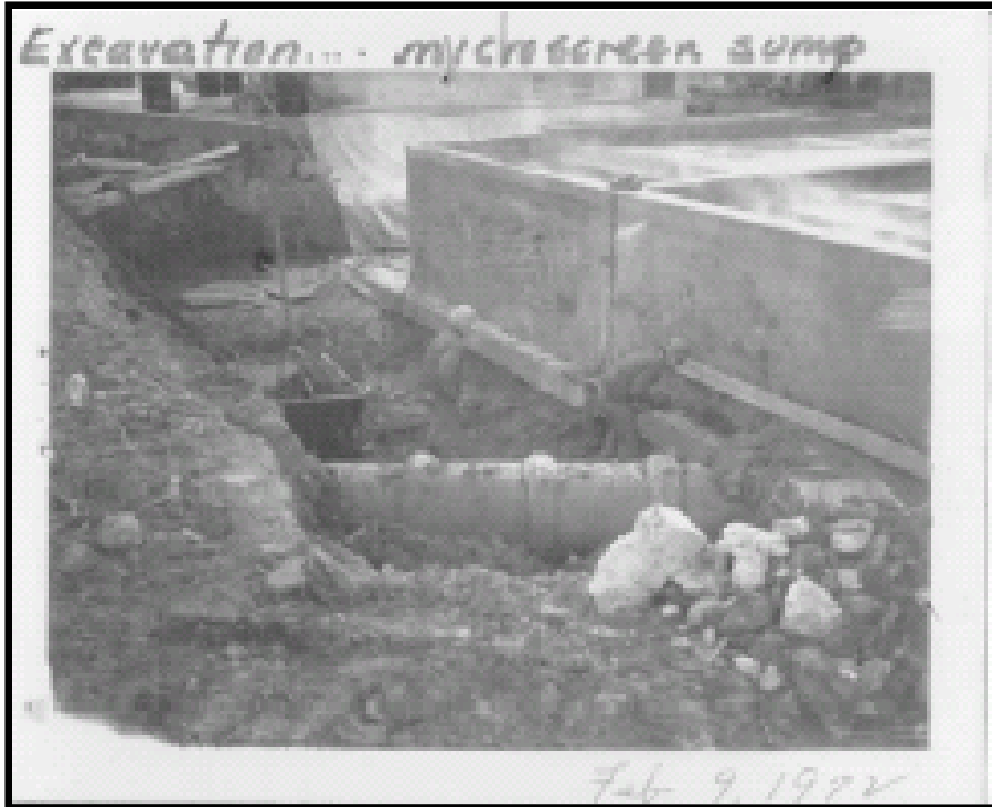
Photo 5 – February 9, 1972 photo. View looking southwest along east side of new settling basins. Note large 30" diameter stormwater pipe in foreground.
