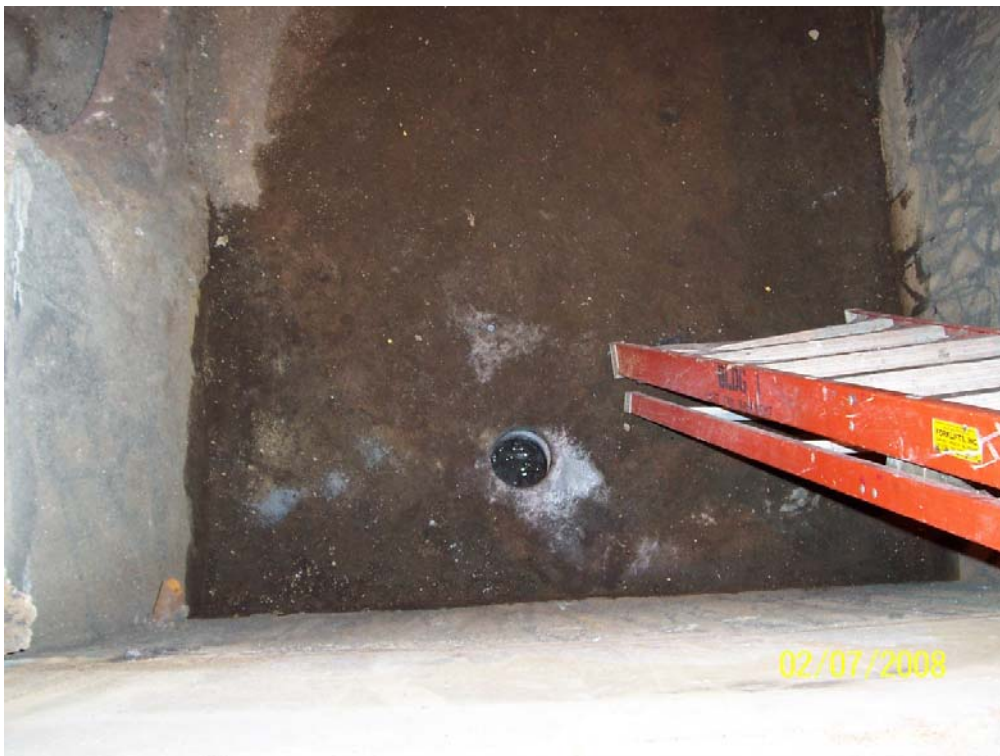
Photo 6 - Building 41, Soil boring 011 with black liquid in crushed stone sub-base.
